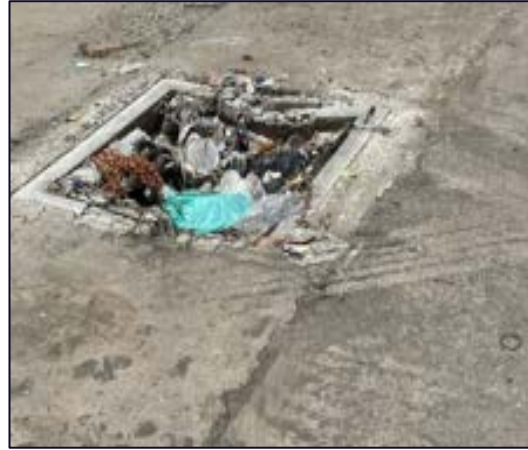
Drainage blocked by plastic waste
