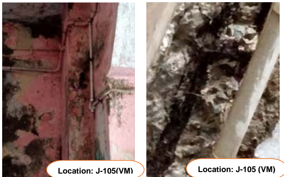
Fig. 8.4: Dampness and Seepage in Vegetable Market.
