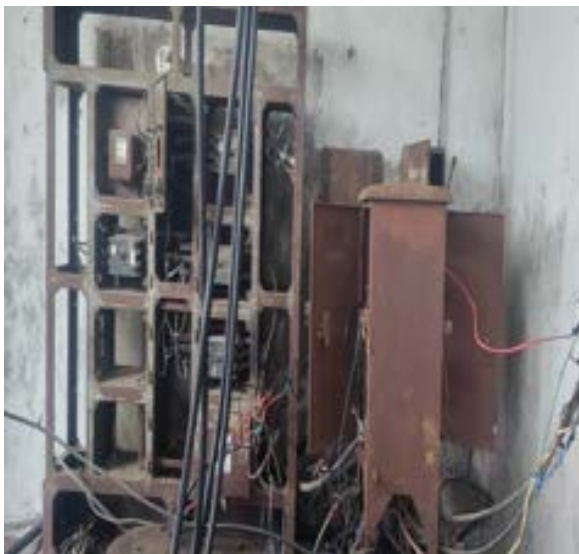
Damaged power line connections
