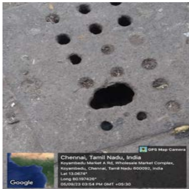
Damaged drainage junctions
