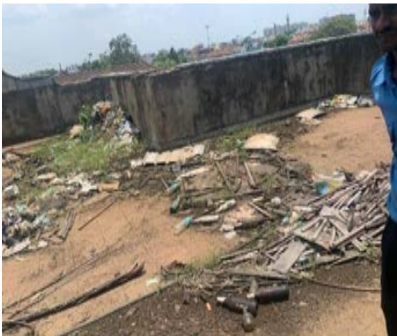
Terrace areas debris blocking rainwater
