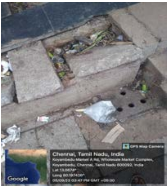
Drainage blocked by solid waste
