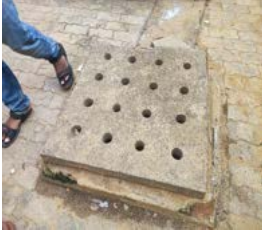
Strom Water Drainage
