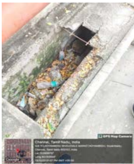
Fig. 7.3: Clogged drain in Food & Grain Market
