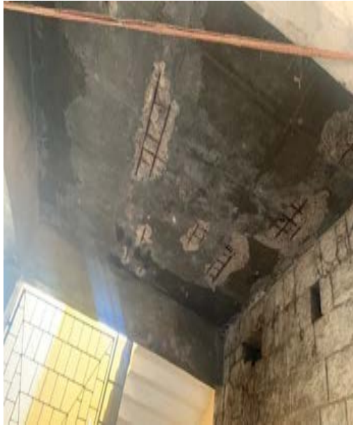
Shop ceiling- spalled / corroded rebar
