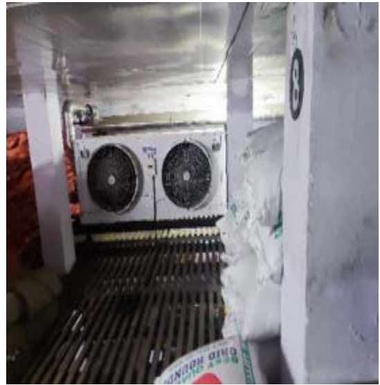
Cold storage room
