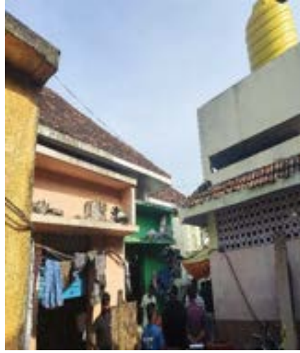
Damaged toilet complex roofs
