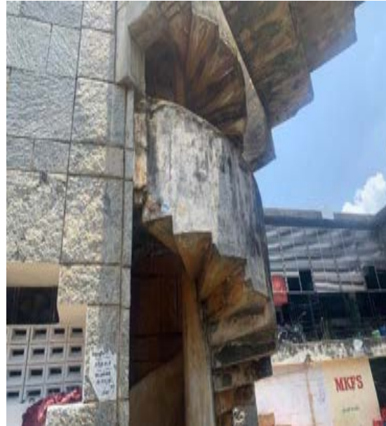
External staircase cracks / damages
