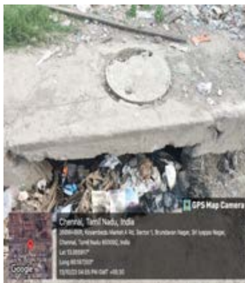
Fig. 7.4: Clogged drain outside Vegetable Market
