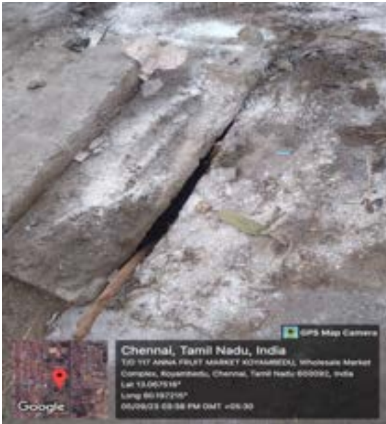
Damaged Drainage slabs
