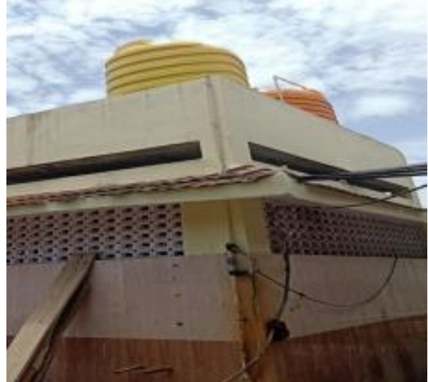
Storage tank provision for each toilet
