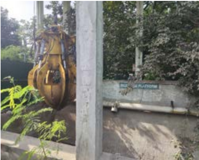
Non-functional Bio methanation plant
