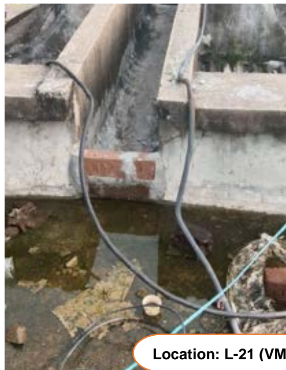
Fig. 8.6: Deterioration of the roof structure
