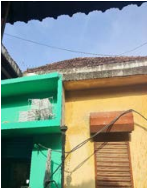
Seepage of water from roof
