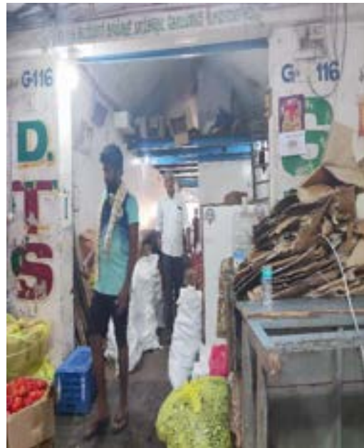
Damage in roof of flower market
