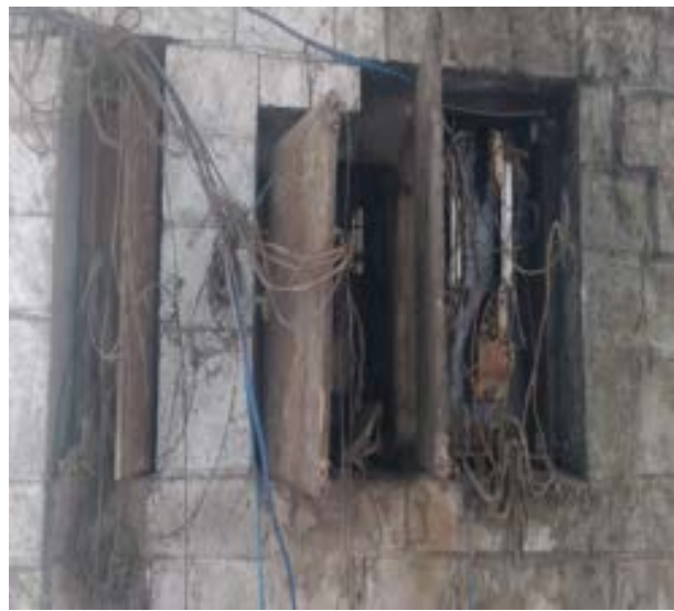
Unmaintained power control boxes
