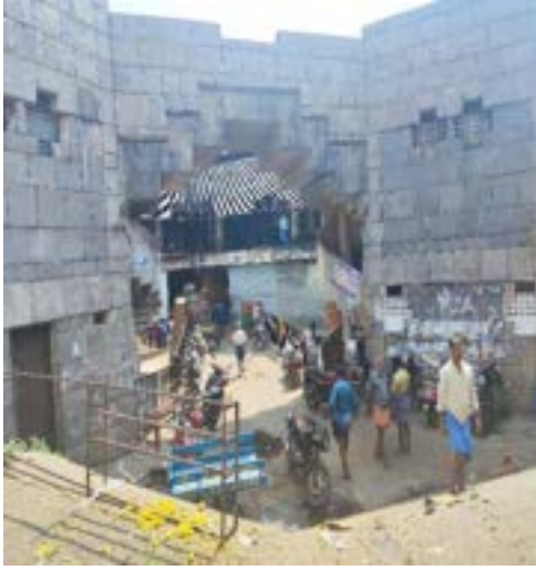
De-structure in the outer walls
