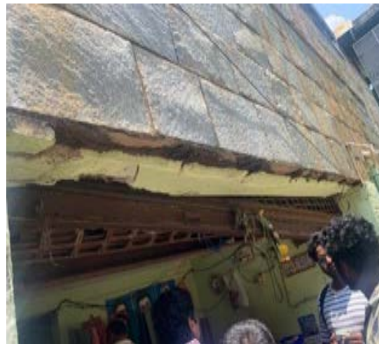
Lintel damage at the shop entrance
