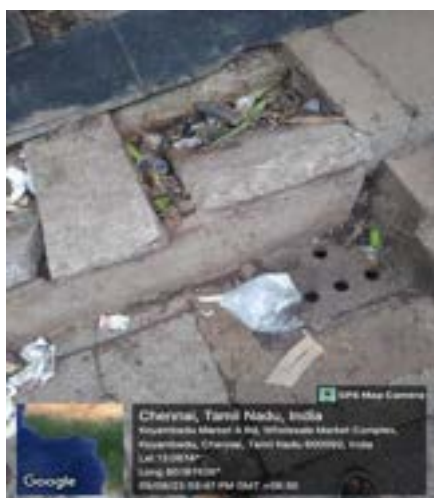
Fig. 7.1: Clogged drain at Fruit market
