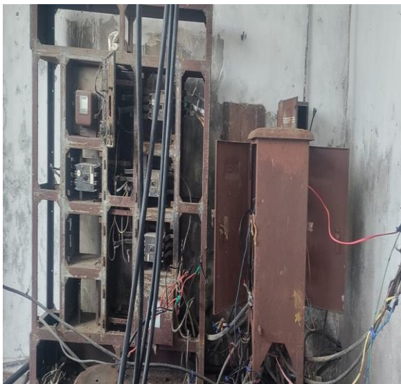
Damaged power line connections
