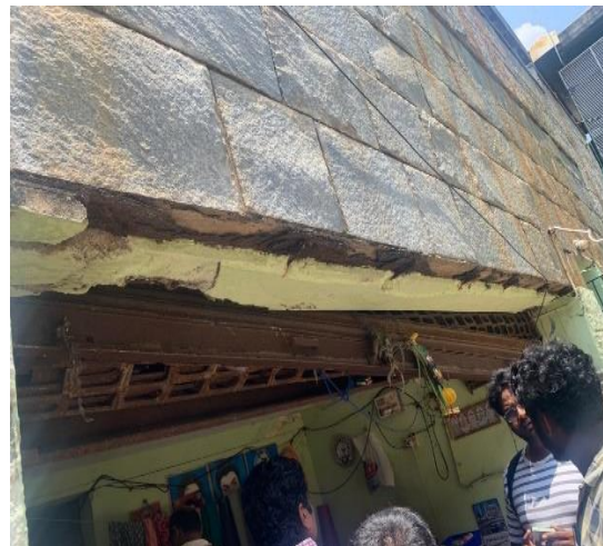
Lintel damage at the shop entrance
