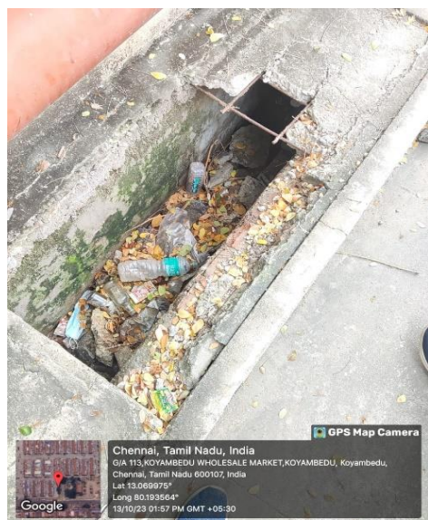
Fig. 7.3: Clogged drain in Food & Grain Market
