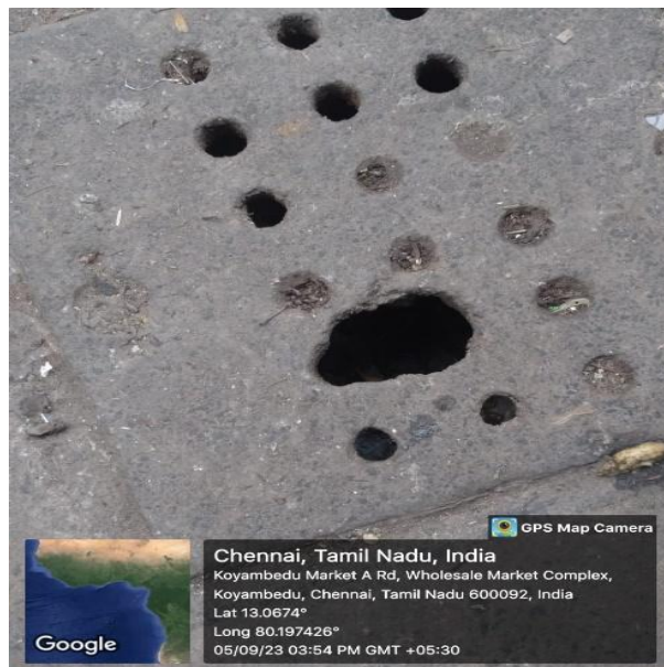
Damaged drainage junctions
