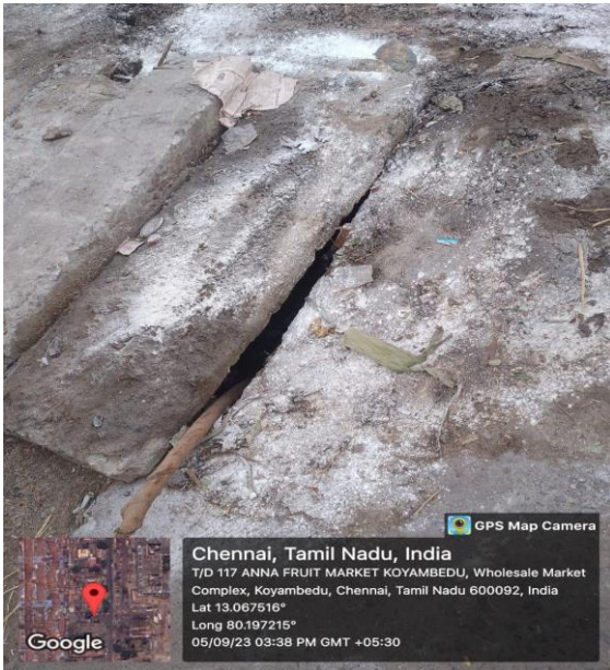
Damaged Drainage slabs
