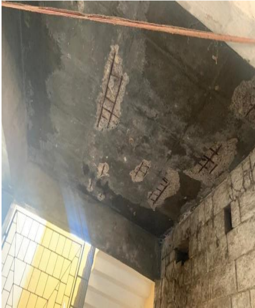
Shop ceiling- spalled / corroded rebar
