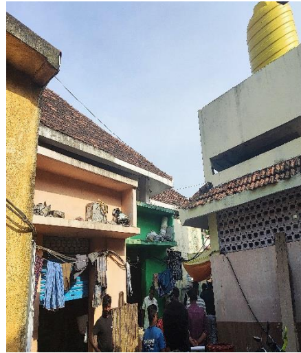
Damaged toilet complex roofs
