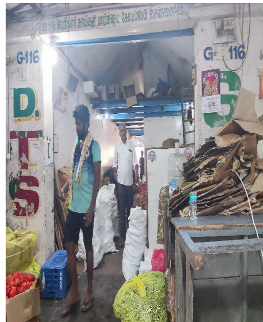
Damage in roof of flower market
