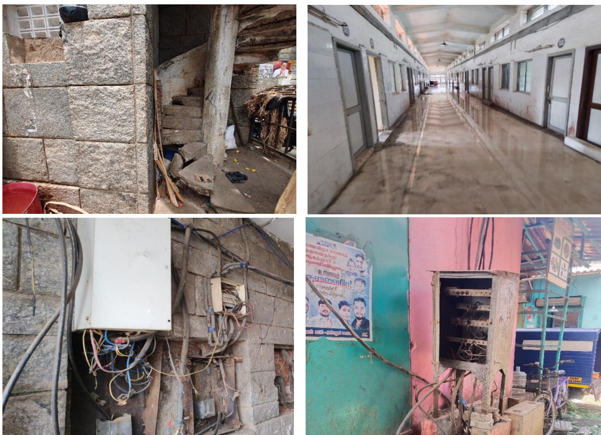
Fig. 11.16: Clock wise from top left: Water seepage issues in grain and flower markets, exposed electricity infrastructure in the veg and flower market
