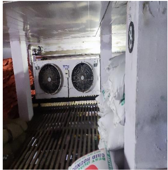
Cold storage room
