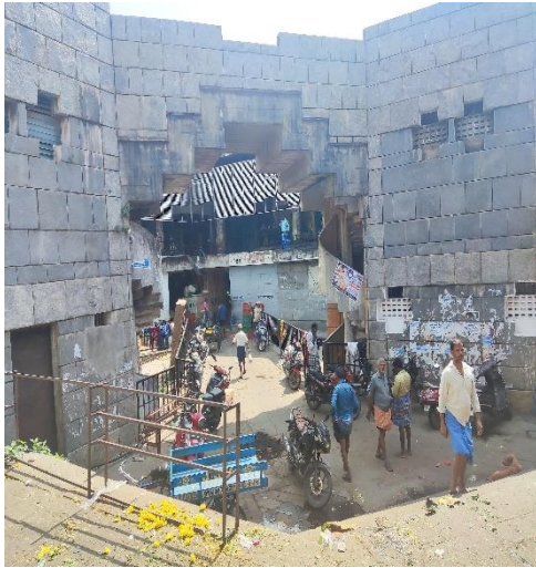
De-structure in the outer walls
