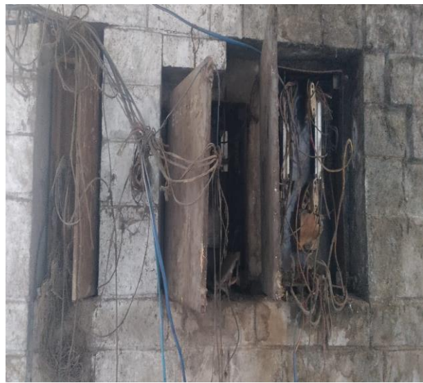
Unmaintained power control boxes
