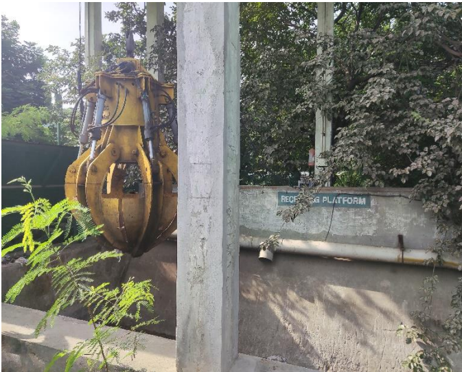
Non-functional Bio methanation plant
