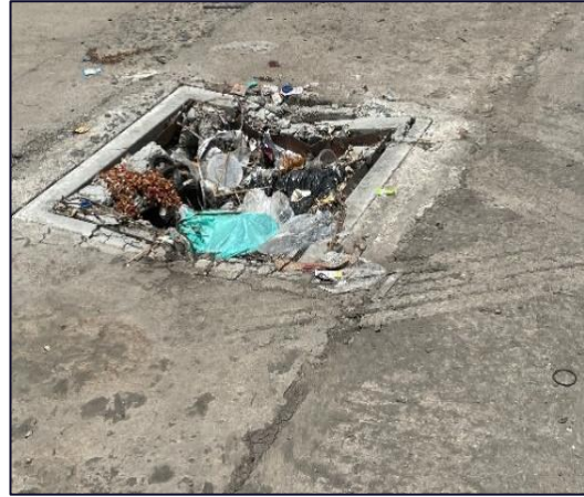
Drainage blocked by plastic waste
