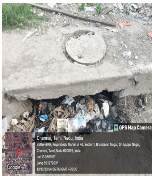
Fig. 7.4: Clogged drain outside Vegetable Market
