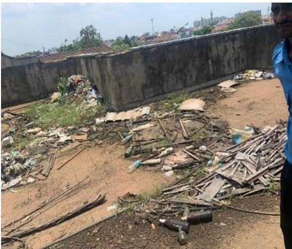
Terrace areas debris blocking rainwater
