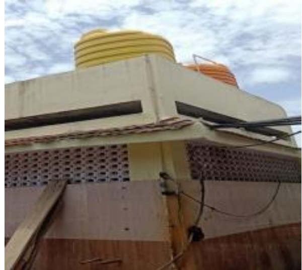
Storage tank provision for each toilet
