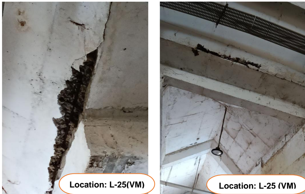
Fig. 8.3: Spalling of Concrete & Loss of Reinforcement
