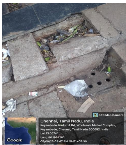
Fig. 7.1: Clogged drain at Fruit market
