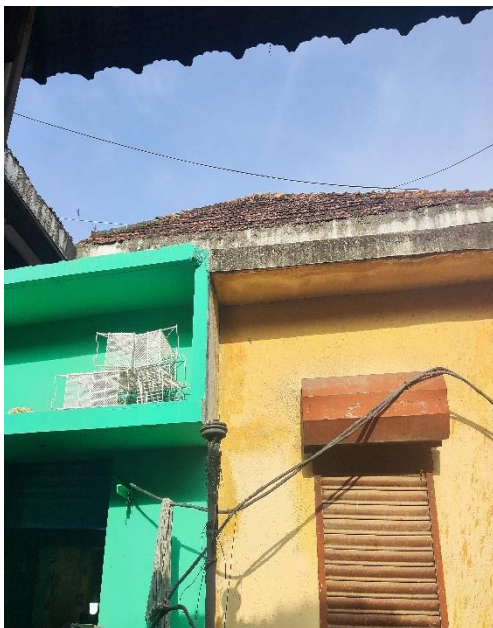
Seepage of water from roof
