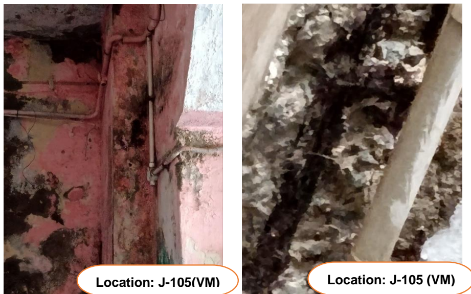
Fig. 8.4: Dampness and Seepage in Vegetable Market.
