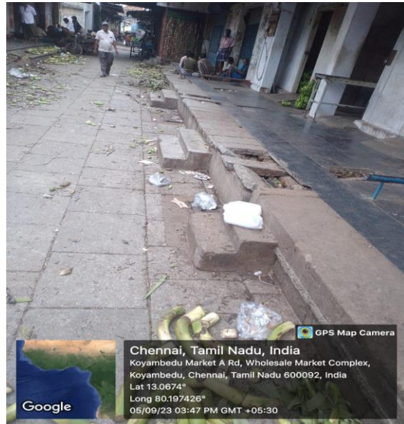
Drainage space occupied by shopkeepers
