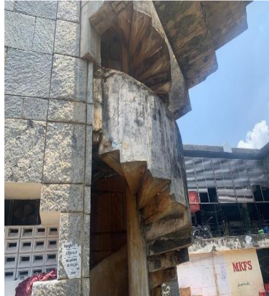
External staircase cracks / damages
