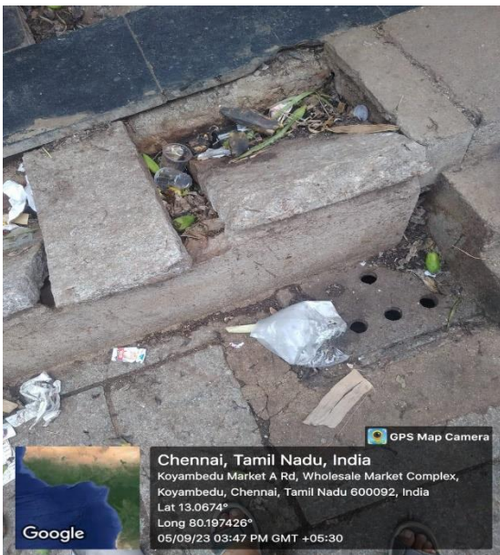
Drainage blocked by solid waste
